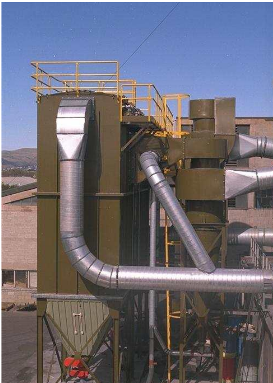
AW Frazer high temperature smelter baghouses complete with grit arrestor
