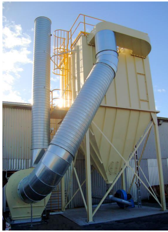
James Hardie Cement fibre board dust Pulse Jet Filters, complete with low pressure blowline
