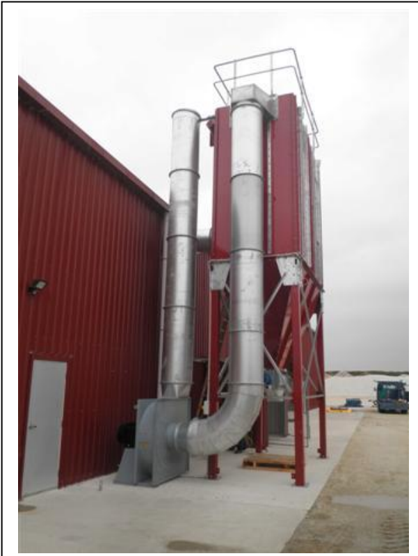
Southern Stone mineral dust Pulse Jet Filter, complete with rotary valve discharge into a skip
